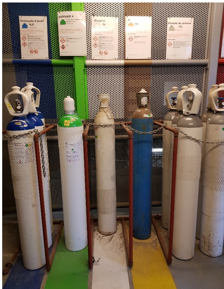
Fig. 2 — A visible identification of the cylinders via clear labeling on the wall and via a color-coded marking on the ground.
