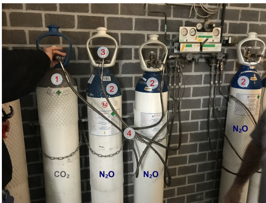
Fig. 1 — CO 2 cylinder (grey shoulder) mistakenly connected to the N 2 O manifold (N 2 O cylinders with blue shoulders). Photo taken by the technician during his checkup of the gas delivery system. 1: CO 2 cylinder, 2: N 2 O cylinders, 3: connection of the fitting on the thread, 4: connecting lines.
